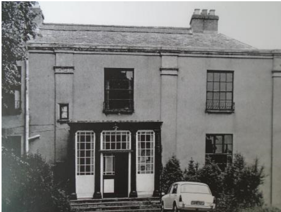
The entrance front c.1970, disfigured with a waste pipe and other alterations. SWHT
